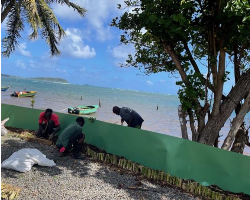
Figure 7 A solid barrier shielding newly planted vetiver in Soubise from the harsh winds & salt spray. Naupaka planted on the sea side will create a top line of protection. When the vetiver grows it will obscure the fence.
